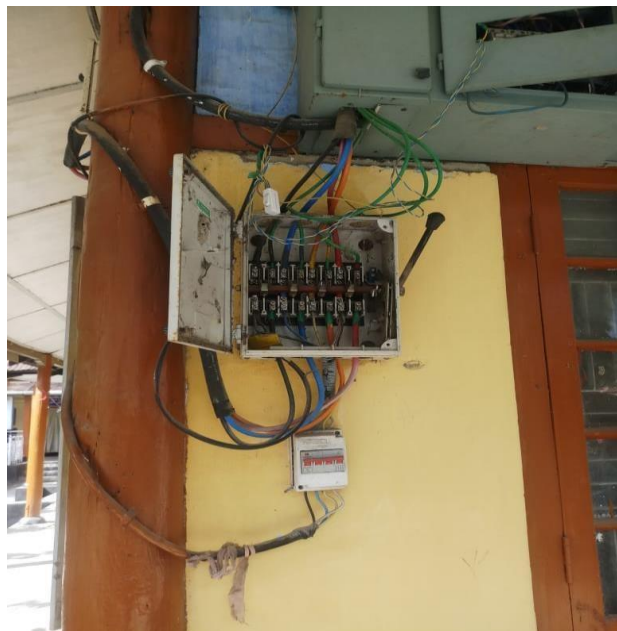
Figure 10: Alternating current obtained from Roof Top Solar Plant is directly interfaced with APDCL supply contributing to energy demand of the college during daytime/solar generation period and thereby reducing overall consumption from APDCL.
