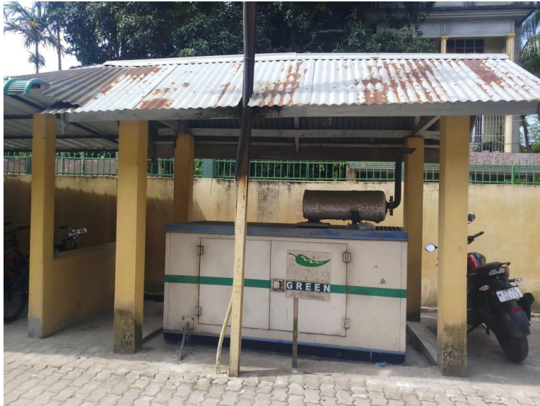
Figure 3: Diesel Generator (DG)
