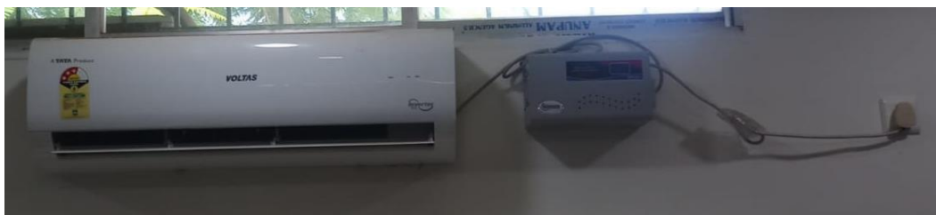
Figure 4: Air Conditioner (AC)
