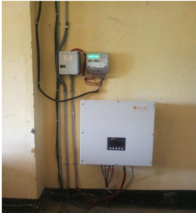
Figure 9: Solar Inverter system for interfacing of ON-GRID 20kWp Solar Roof Top system with APDCL mains. DC generated from solar panels converted to AC for usage.
